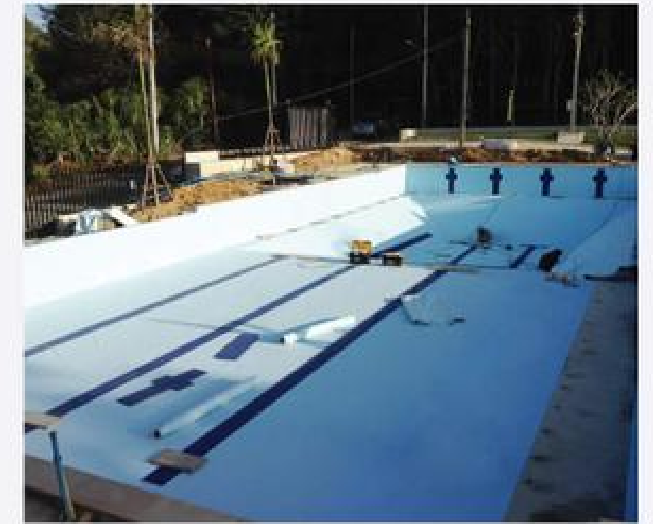
Liner Pool No leaking 100%
